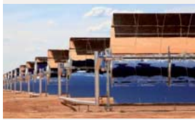
Iberdrola Renovables' first solar thermal plant.
