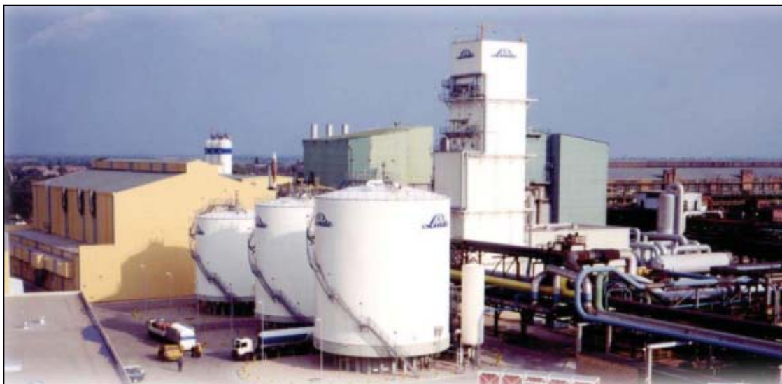
This cryogenic air separation unit at the Leuna refinery produces 1,500 tons/day of gaseous oxygen and 2,700 tons/day of nitrogen, plus 400 tons/day of liquid oxygen, nitrogen, and argon (Fig. 3).
