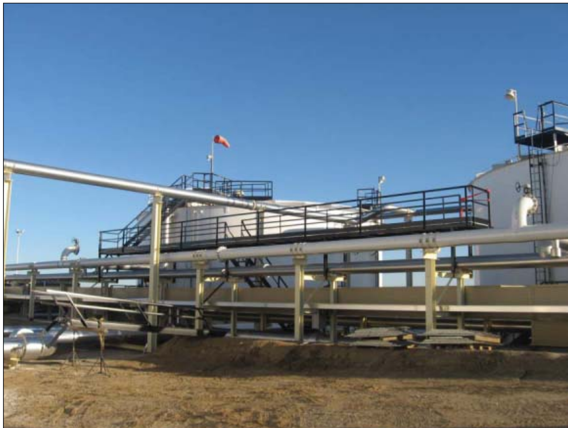
The project included the installation of several access platforms on the six tanks (Fig. 5).
