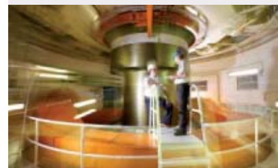
Itaipu hydroelectric dam, Brazil.
