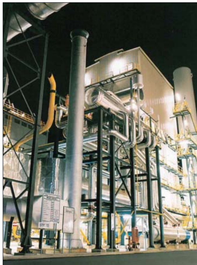
Here is an example of a steam reformer, in the Milazzo refinery, Sicily (Fig. 1).
